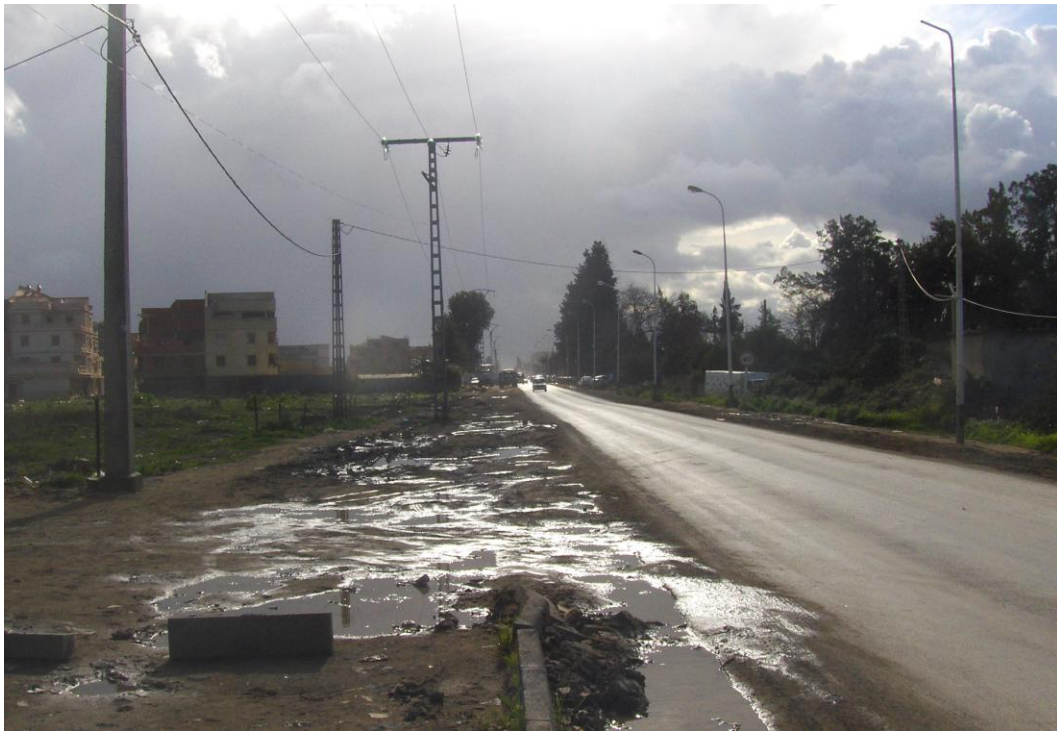
Fig. 4 – Pavements with little or no maintenance. Cherarba, along the N 61.
